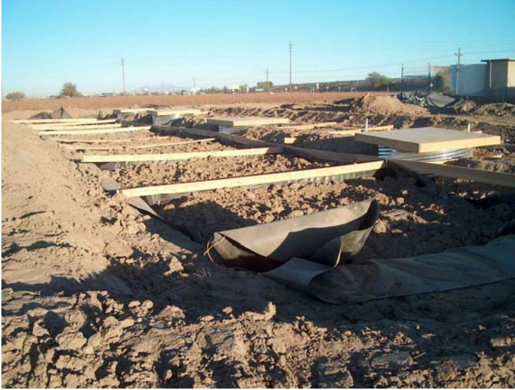
Photo 5 - View looking north of the lined and backfilled halophyte plots. Salt tolerant plants will be planted on top of the soil.
