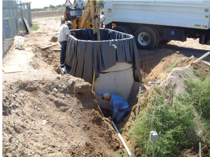
Photo 6 – Replacement slow sand filter being installed. As shown, one sand filter is concrete. Another sand filter, not shown, is semi-buried with liner and framing.
