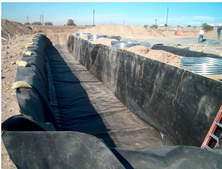
Photo 3 - 40-mil HDPE liner installed for halophyte plot. Over 3,800 square feet of liner was used for each of the two plots.
