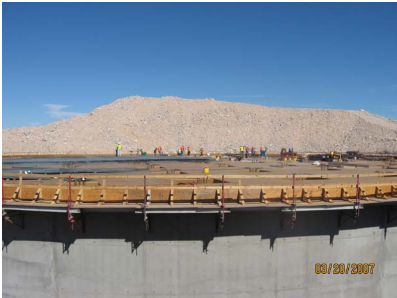
Workers are finishing the temporary roof deck of the Northeast Reservoir. A steel reinforced concrete roof will be placed on the deck and the decking will then be removed. Once the roof has been completed, the large mound of dirt pictured in the background will be placed around and on top of the reservoir. Natural vegetation will be planted on top of the reservoir so as to make the reservoir completely unnoticeable under its desert landscape.
