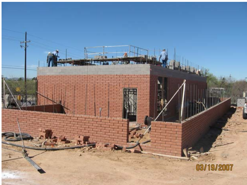
The Northeast Reservoir Booster Station, located on Magee Road near La Canada, will pump water into the distribution system and fill the Northeast Reservoir.
