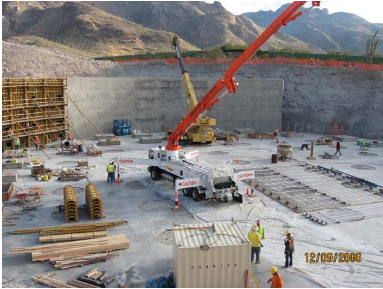
After the steel reinforced concrete flooring was completed on the Northeast Reservoir, construction crews began to erect the walls.
