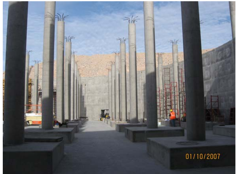
Concrete columns to support the roof of the reservoir were placed on the floor of the reservoir.
