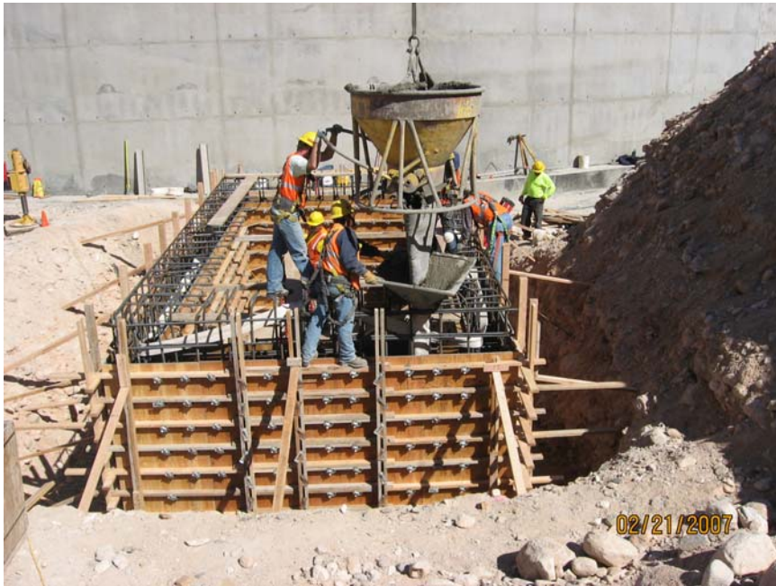
Underground vault next to the Northeast Reservoir will house inlet and outflow flow control valves.
